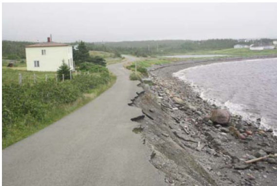
Figure 32. Coastal erosion at Admiral’s Beach, Avalon Peninsula, undercut this transportation route. Source: Batterson and Liverman, 2010 181
